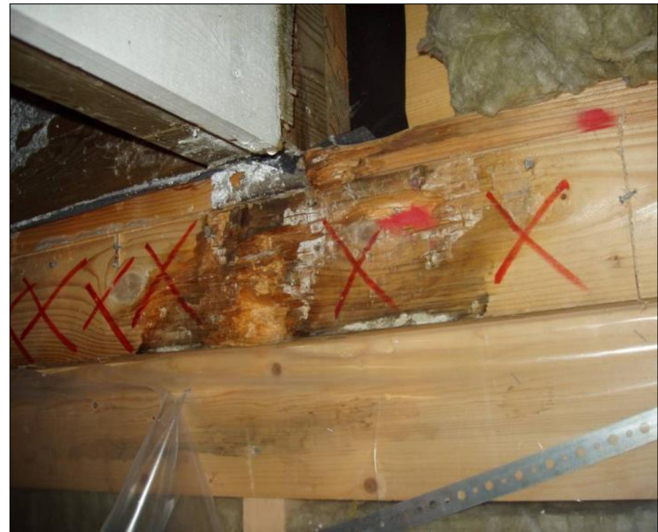
Rot in a load-bearing beam after two years
