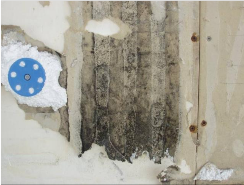
Mould growth on the exterior gypsum board
