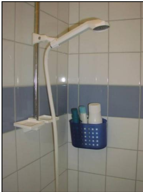
Wet room wall behind tile
