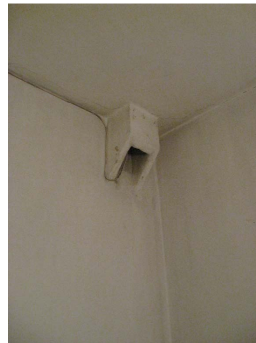
District Heating Exhaust hood in kitchen
