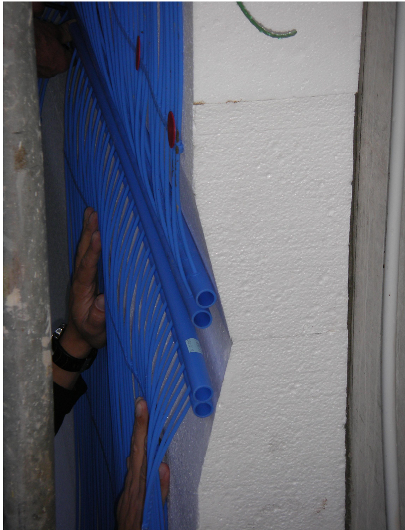
Cutting out of the insulation board for the integration of the collecting pipes
