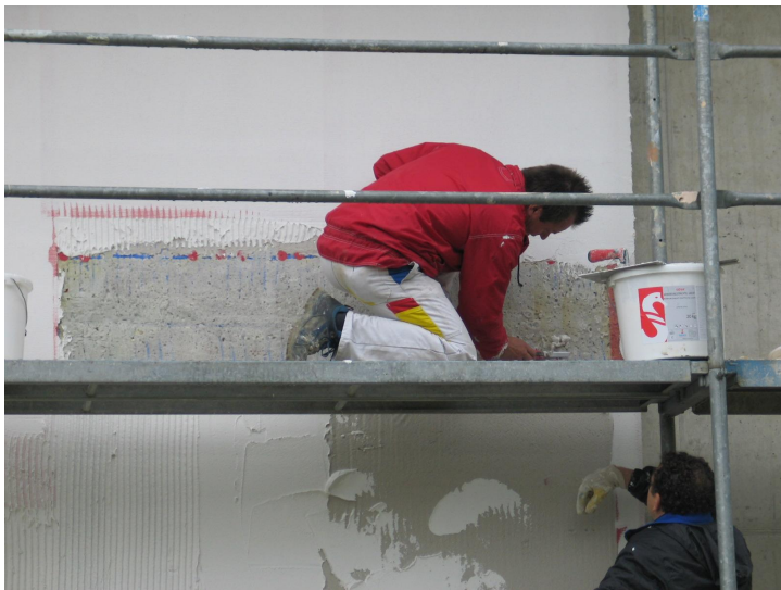
Application of the organic under coat and integration of the reinforcement fabric
